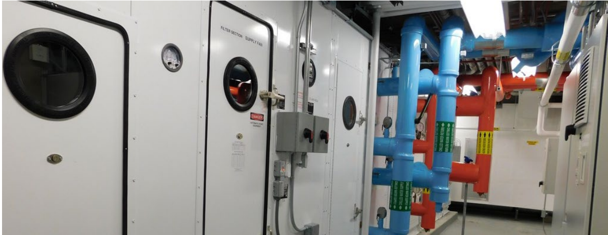
Physical Science II Building - Air Handling Unit #2
